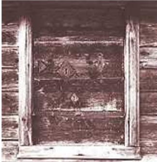
Illustration 1: The seven locks on the grain store door illustrate in-depth knowledge of forging techniques.
